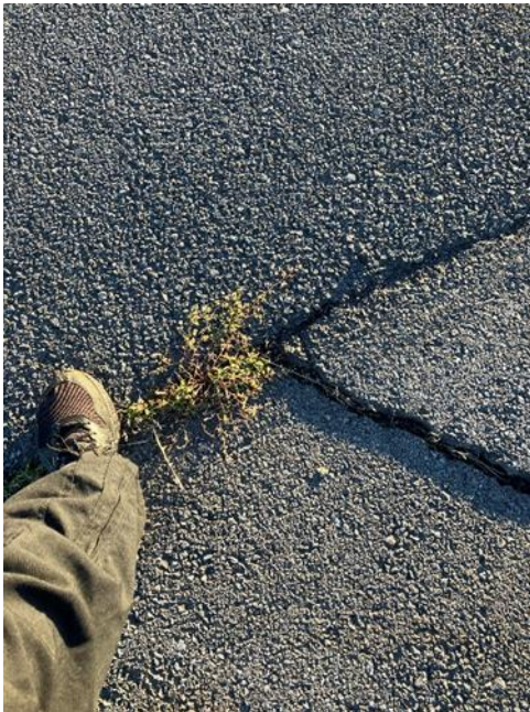
Runway 1 Asphalt Distress
