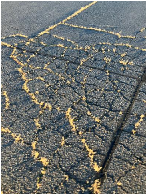
Apron 3 Asphalt Distress
