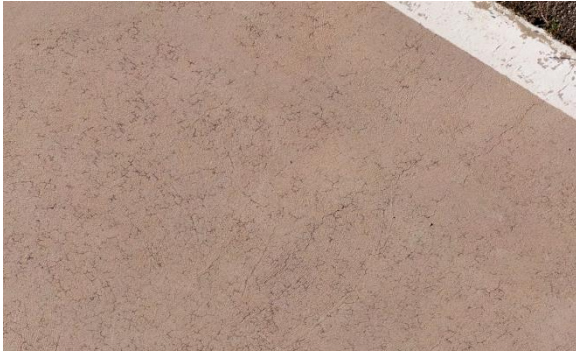
19) 73 – Shrinkage Cracking, Asphalt – Section H1A
