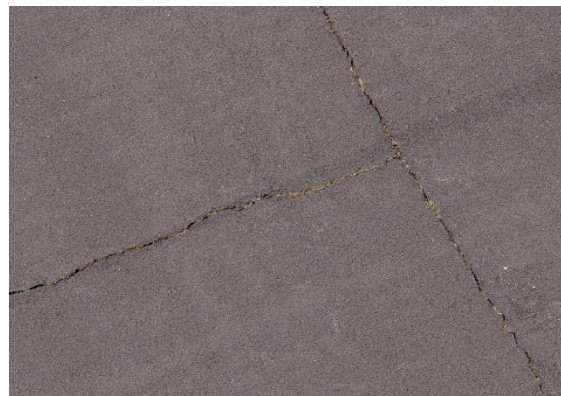
6) 48 – Longitudinal and Transverse Cracking Medium, Asphalt – Section A1
