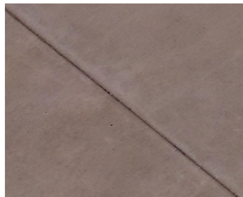
12) 65 – Joint Seal Damage Low, Concrete – Section H2
