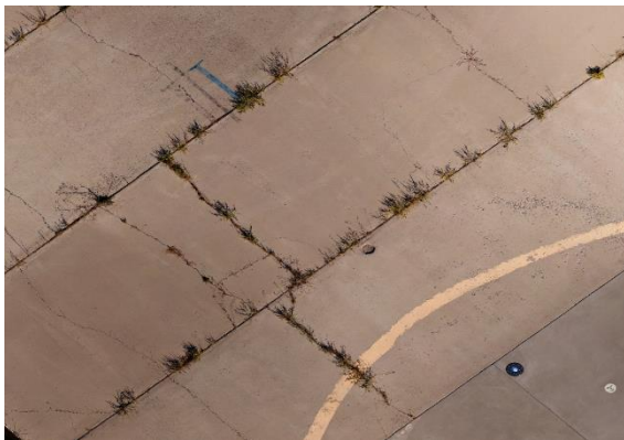
17) 72 – Shattered Slab Medium, Concrete – Section H2
