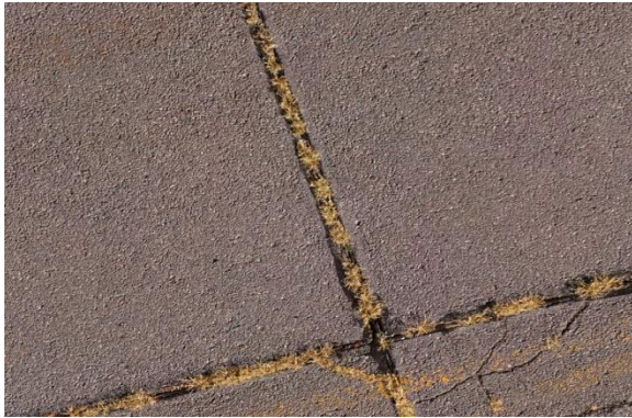
3) 47 – Joint Reflection Cracking Medium, Asphalt – Section TD1
