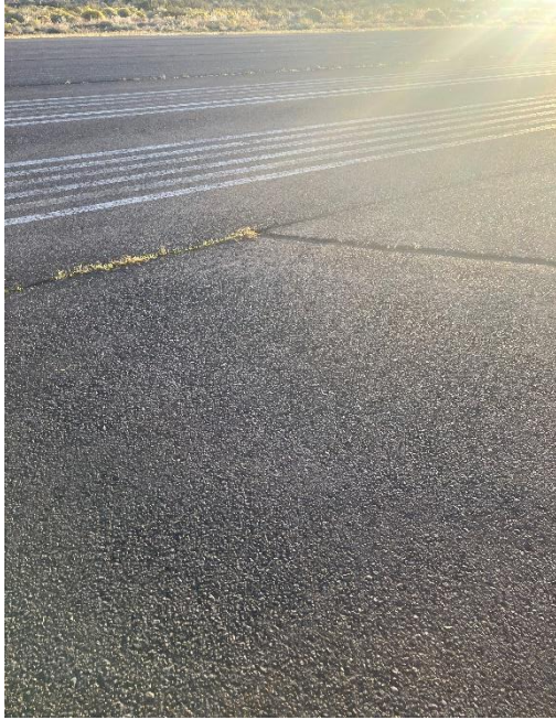
Runway 3 Asphalt Distress
