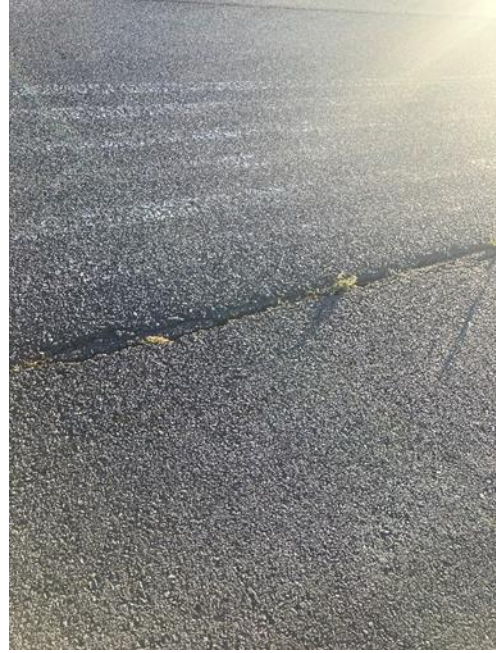
Runway 4 Asphalt Distress
