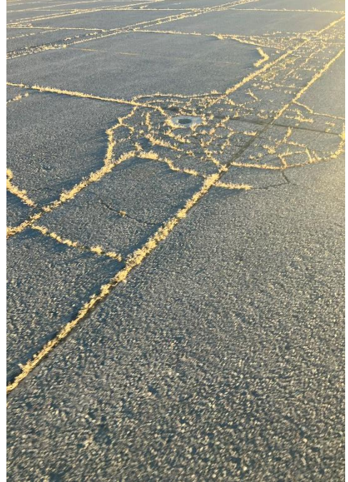
Apron 2 Asphalt Distress
