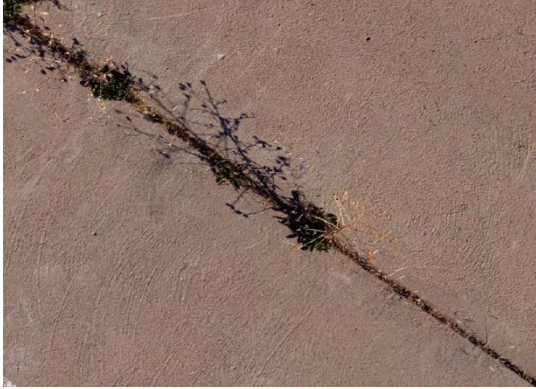
13) 65 – Joint Seal Damage Medium, Concrete – Section H1A
