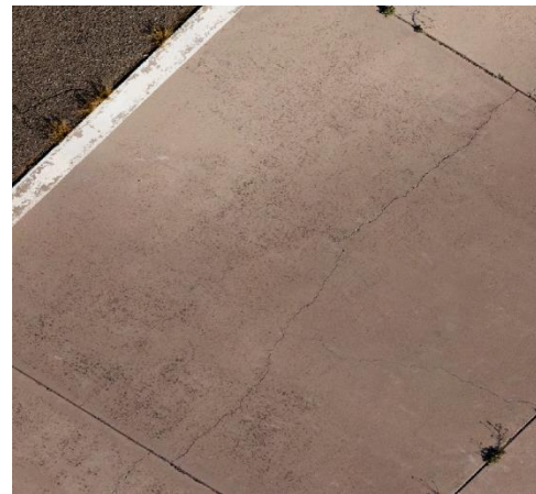
10) 63 – Longitudinal, Transverse, and Diagonal Cracking Low, Asphalt – Section H1A
