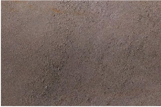
7) 52 – Raveling Low, Asphalt – Section TD1
