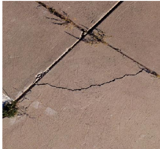
21) 75 – Corner Spalling Low, Concrete – Section H1A
