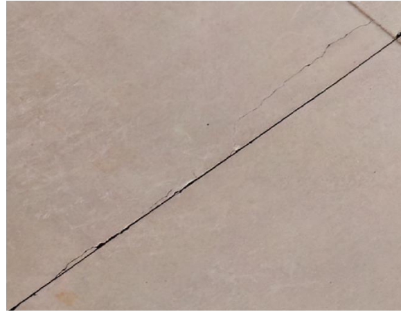
20) 74 – Spalling Longitudinal and Transverse Joint Low, Concrete – Section H2
