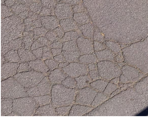
1) 41 – Alligator Cracking Medium, Asphalt – Section A1
