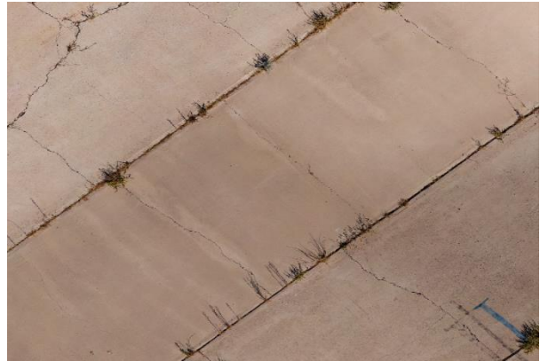
16) 72 – Shattered Slab Low, Concrete – Section H2
