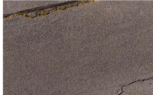
8) 52 – Raveling Medium, Asphalt – Section TD1
