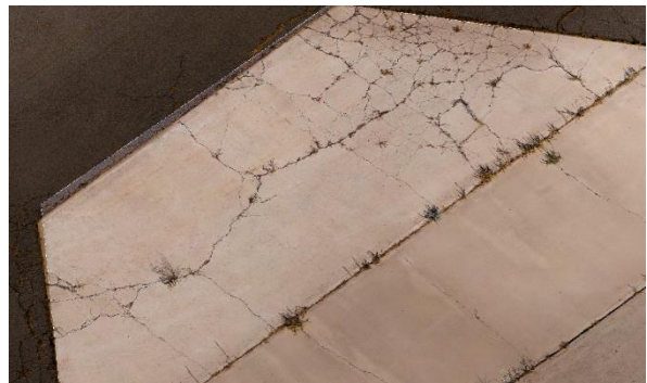
18) 72 – Shattered Slab High, Concrete – Section H2
