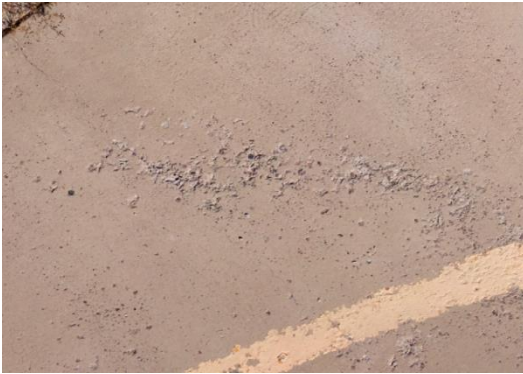
15) 70 – Scaling Medium, Concrete – Section H2
