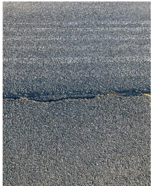
Runway 2 Asphalt Distress
