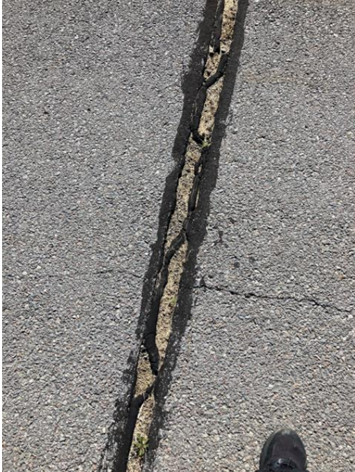
Apron 5 Asphalt Distress
