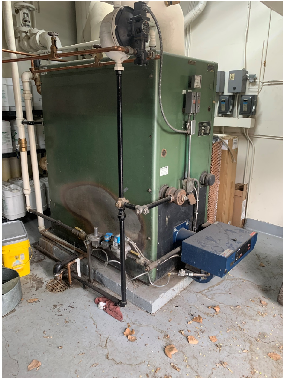
Figure 1 – Existing Heating Water Boiler
